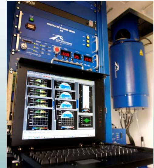
View inside the Lidar shelter: electronics rack with operator GUI (left) and laser unit (right)
